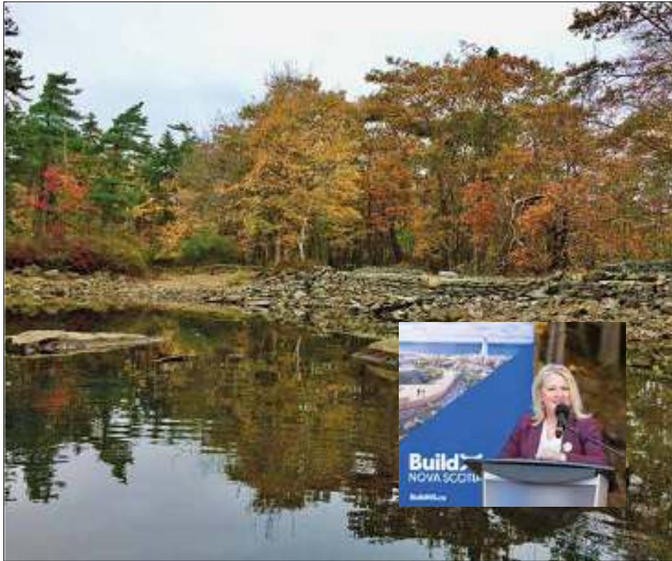
Deteriorating Williams Lake Dam to be rebuilt by Build Nova Scotia, Shaw Wilderness Park. Photo of dam: Cathy Vaughan, October 2021
