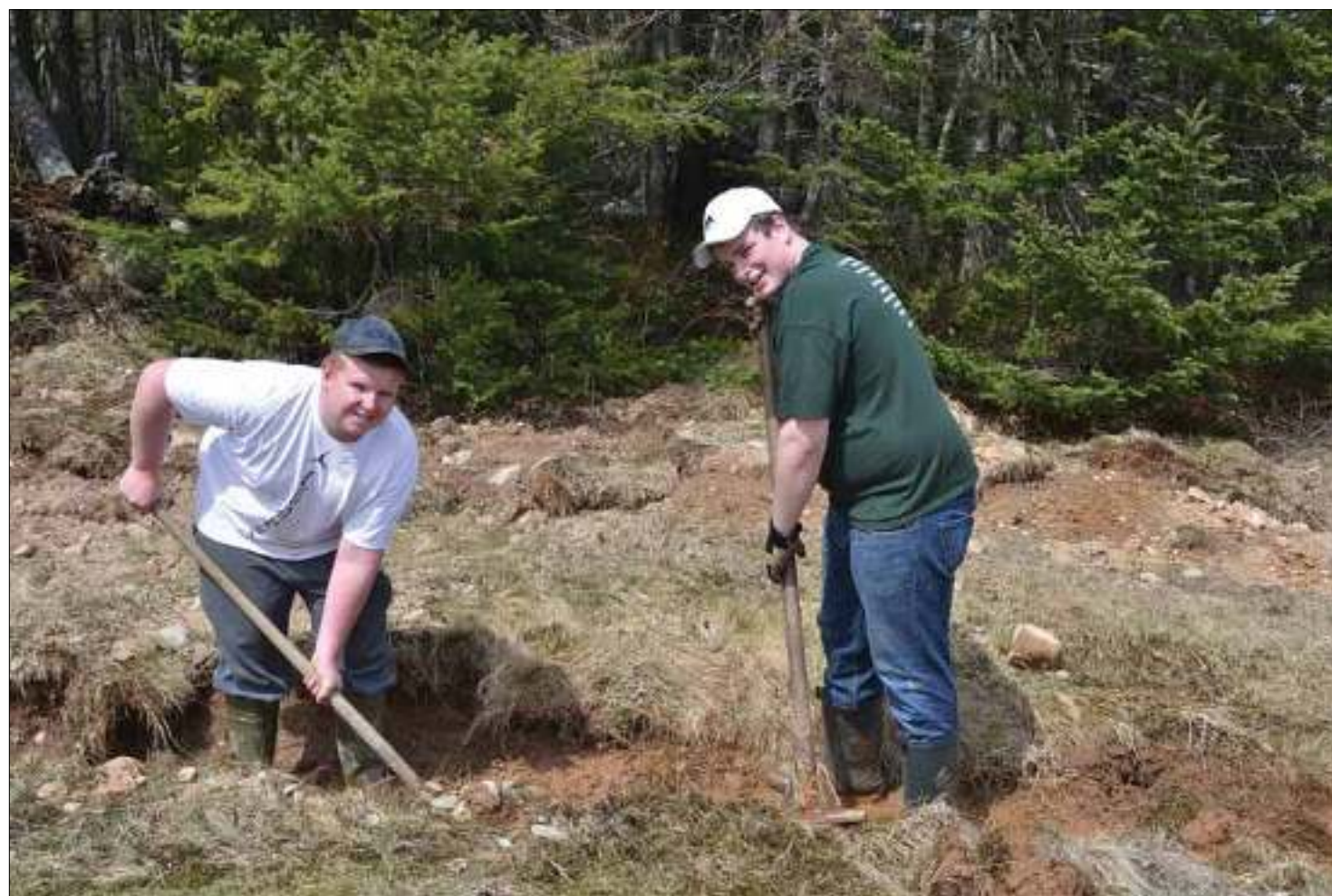
Ryan and Joseph have been busy working on improving drainage on the course
