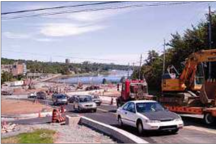
Construction at the Armdale Rotary is behind schedule a couple of weeks, mainly due to workers uncovering unknown infrastructure. But officials are aware that September is here and have made plans to keep traffic lanes open during peak morning and afternoon rush hours.
