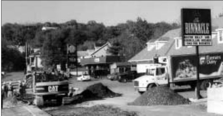
Sidewalk construction on this section of Purcell's Cove Road caused a stir between the city and local businesses which felt the timing of the project was inappropriate.
